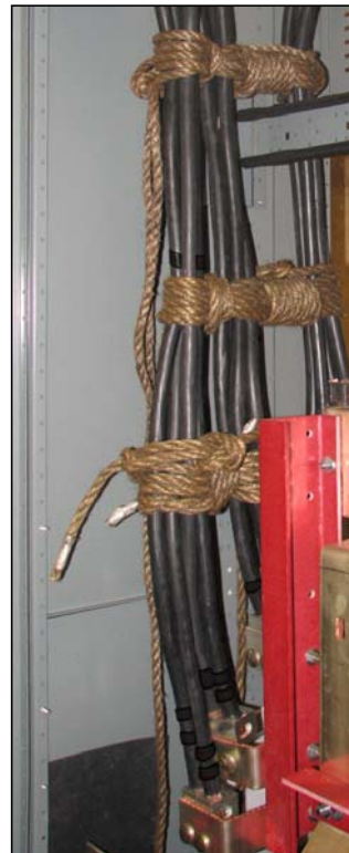
Figure 24 – Cable Restraint Example
