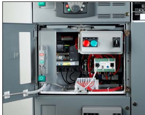
Figure 120: Handles Flush with the Front of the MCC
