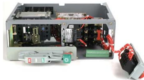
Figure 86: Control Station Plate Removed
