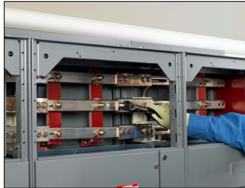
Figure 36: Removing the Left Bolts and Loosening the Right Bolts on the Splice Assembly
