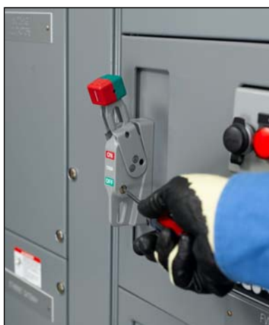
Figure 97: Operating Door Interlock Defeat Mechanism
