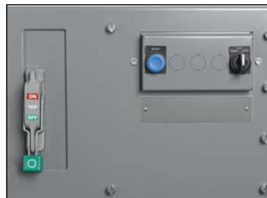
Figure 74: Arc-Rated MCC Door Latches
