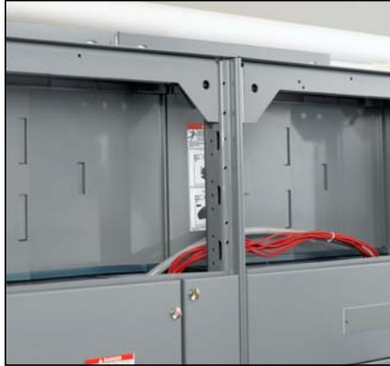
Figure 61: Wiring in the Top Horizontal Wire Trough
