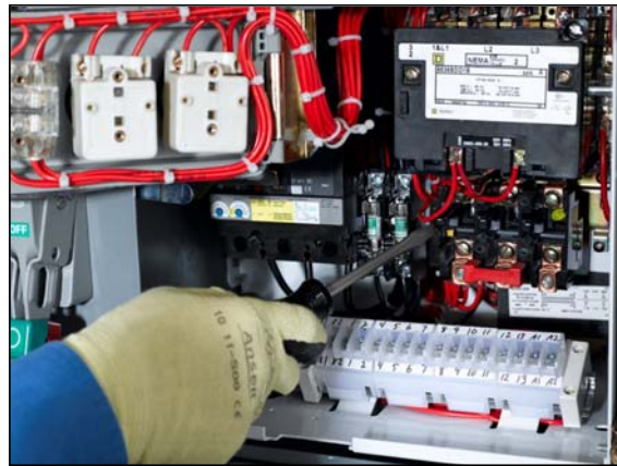
Figure 93: Tripping the Overload Relay
