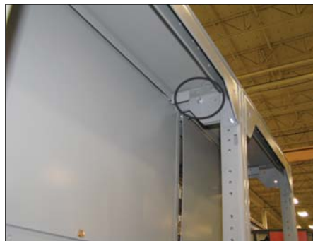
11G: Top Rear Side Channel Connection (Shown with MCC back plates removed.)
