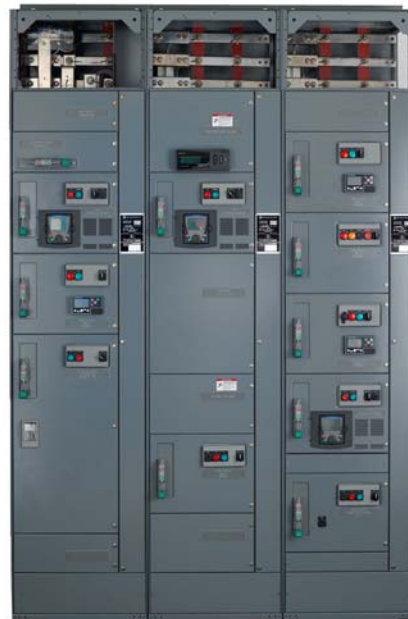
Figure 28: Horizontal Wireway Covers and Bus Barriers Removed
