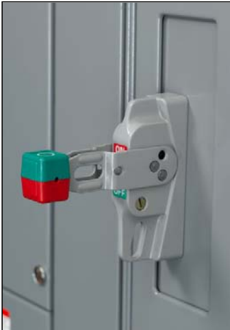
Figure 89: Operator Mechanism in the Tripped Position
