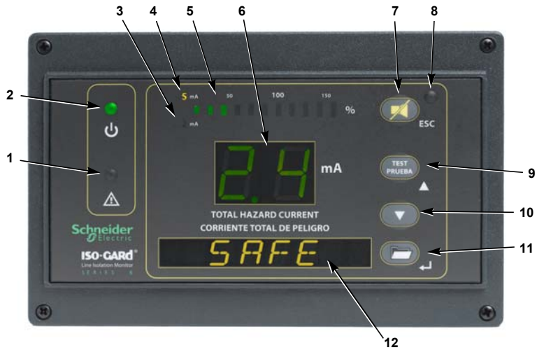
Figure 8: Front Panel Display—Normal Condition
