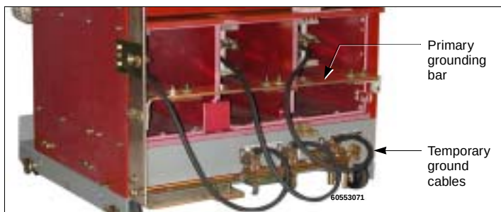
Figure 39: Primary Grounding Bars and Temporary Ground Cables
