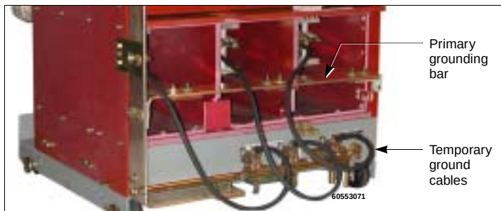
Figure 7: Primary Grounding Bars and Temporary Ground Cables
