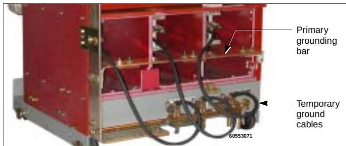
Figure 23: Primary Grounding Bars and Temporary Ground Cables
