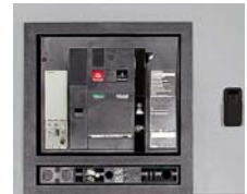
Figure 3: Circuit Breaker Compartment with Secondary Horizontal and Vertical Wireways
