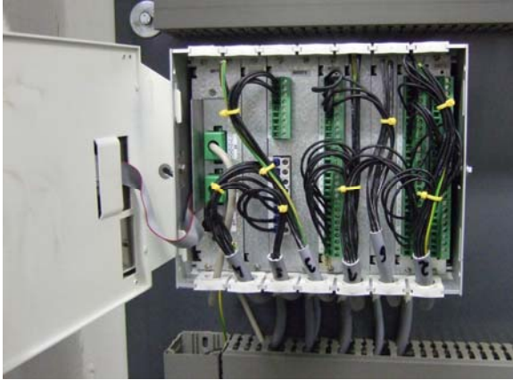
Example of bad cable connection with unnecessary loops (and on top of that there is no functional grounding)
