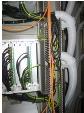
Wrong (unnecessary loops)
