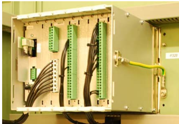
Good connection if paint has been removed properly! However, functional grounding is missing!
