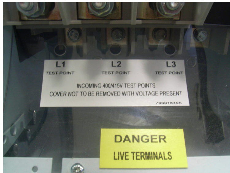
Typical Voltage Test Point Label
