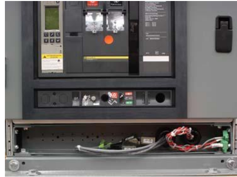
Figure 36: Example of Communication Cables Temporarily Stored in Wireway for Shipment
