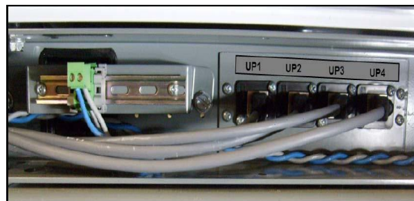
Figure 37: Example of Gray ULP Cables Connected to ULP Ports
