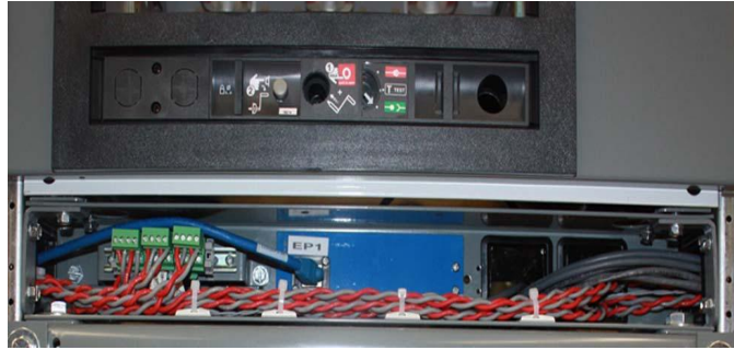
Figure 43: Example of Ethernet Modbus TCP Cable (Blue) Connection to Labeled Ethernet Port
