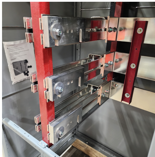
Figure 5 - 4000 A Through Bus Assembly
