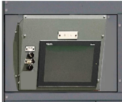
Figure 43 - HMI Touchscreen Shown on Switchboard / Switchgear Door
