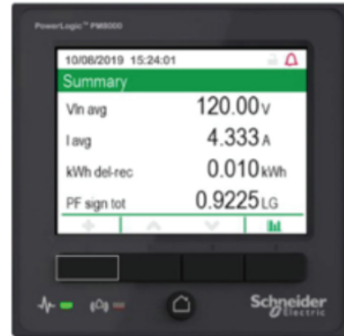
Figure 15 - 3.5 in. Color Graphic Display (mounted on Main Circuit Breaker Door in QED-2)
