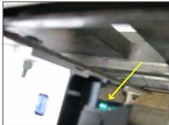
9. Electric arc is visible just when switching ON.
