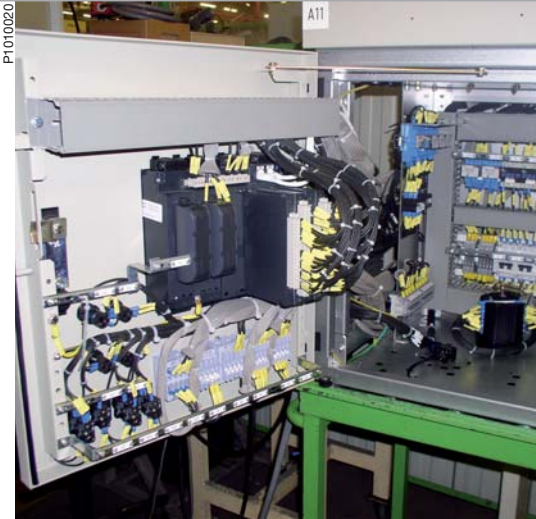
Low voltage compartment
